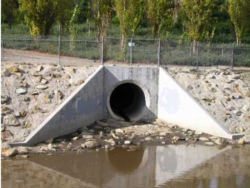
Storm drain system outlet
