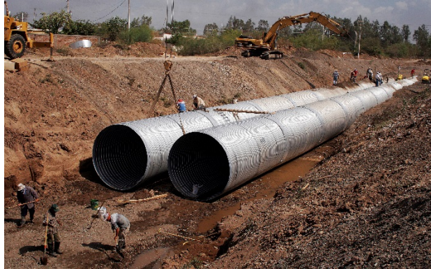
Storm sewer conveyance pipes
