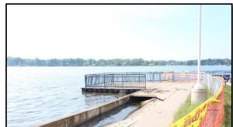
Image: Pathway damage due to high water at Kollen Park in the City of Holland
