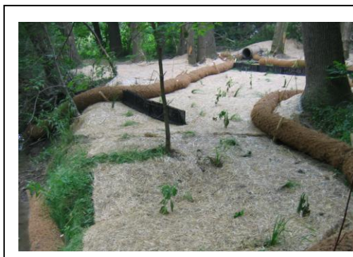
OCRC's newly constructed bioswale along 104 th and James Street and Chicago Drive
