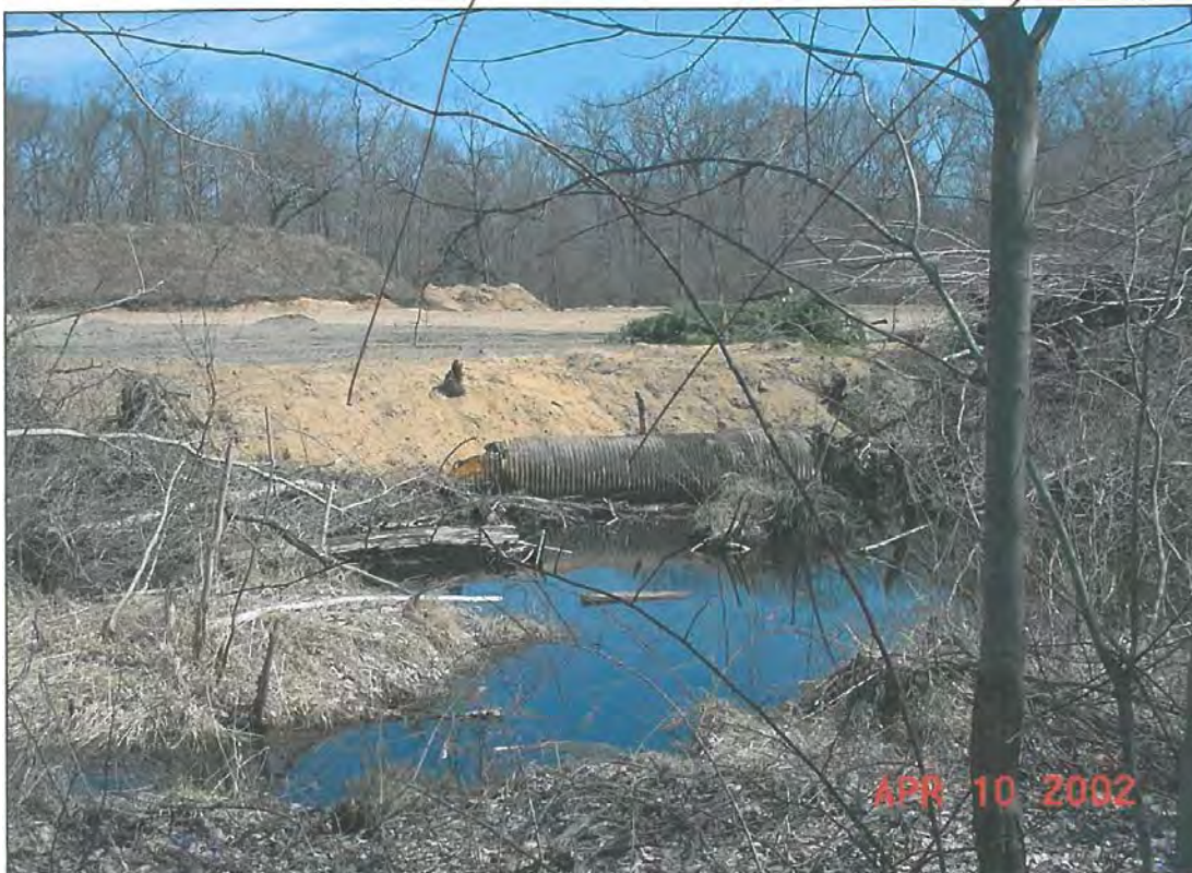
Wetland/shallow pond with outlet to stream. Topsoil storage in distance. Pipe was removed.
