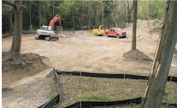
Location: Holland Township, south of Riley, between 104th and 112th. This site is on private property. Please call the MACC to arrange to see it.
