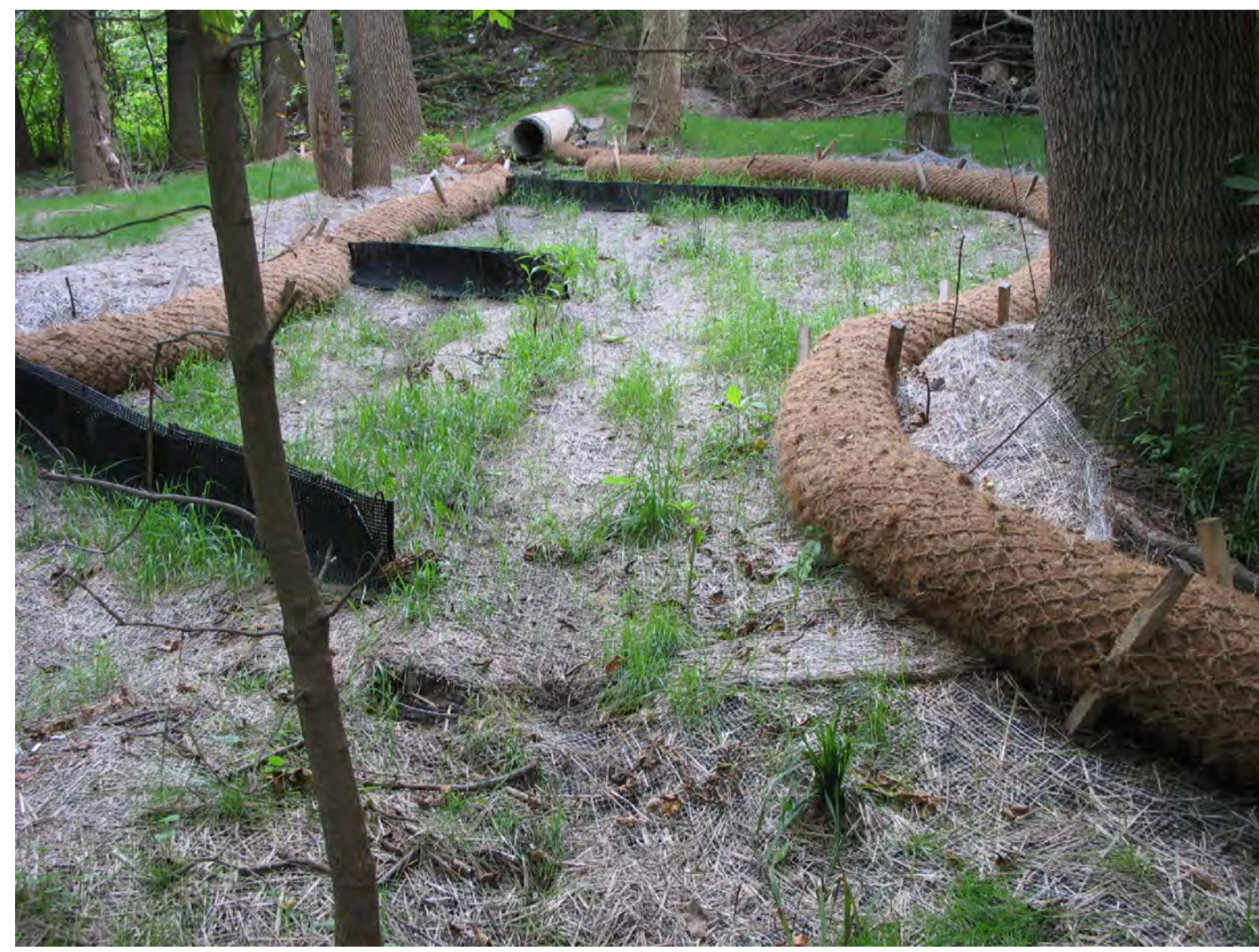
Ottawa County Road Commission Storm Water Outfall Bioswale (2007) Stabilized an area of severe erosion due to a storm water outfall by addition of an infiltration bioswale and coir logs. Supported by OCRC, the Great Lakes Basin Program and the MACC.
