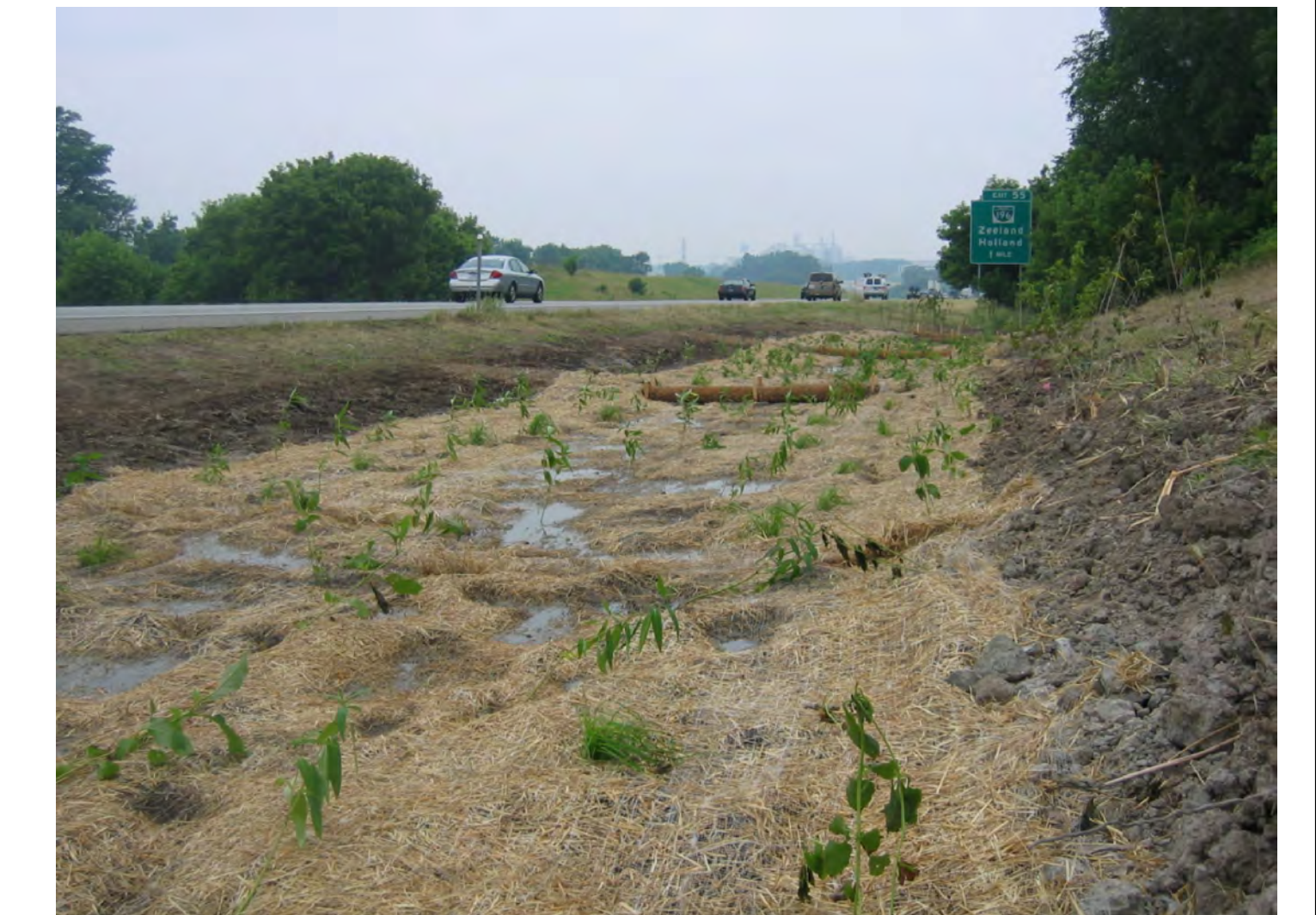
MDOT Roadside Bioswale (2007) Repair of a roadside drainage way to reduce erosion. Supported by MDOT, the Great Lakes Basin Program and the MACC.
