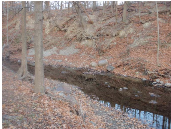
Erosion along Valley Wall downstream of 147th Street
