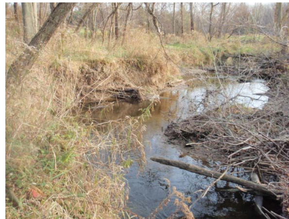
Incised Channel with debris downstream of I-196 BL
